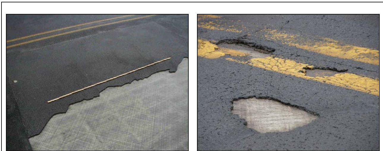
Figure 3. Sections of the polymer concrete wearing surface debonded from the FRP deck. These are photos of Bentley Creek but it has occurred on other bridges as well.
