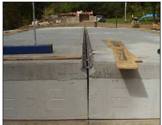
Figure 8. Longitudinal field joint was reinforced with stainless steel reinforcing and grouted with a non-shrink grout.
