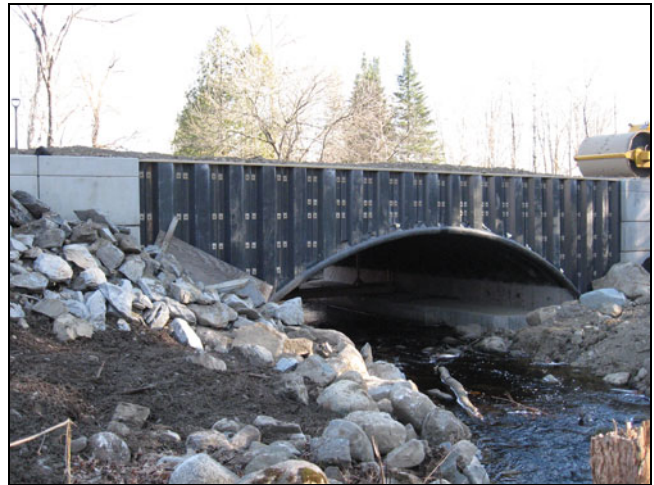
Figure 11. This bridge illustrates Maine's innovative use of composite materials for structural members.
